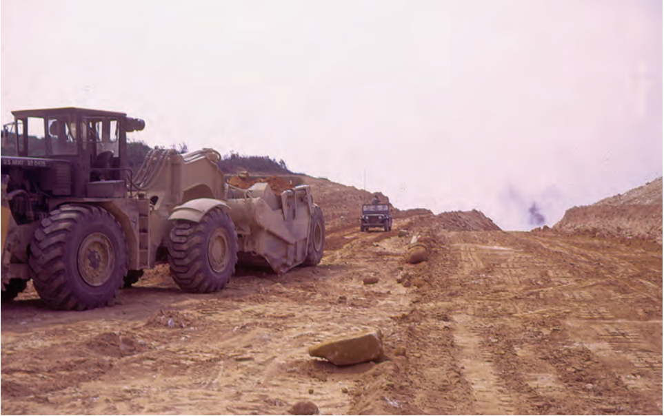
At the top of Hai Van Pass, the 35th Engineer Battalion deployed equipment like this 290M scraper to widen the road and reduce sharp curves.
